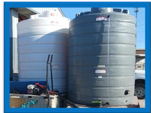
Brine storage station at Public Works
